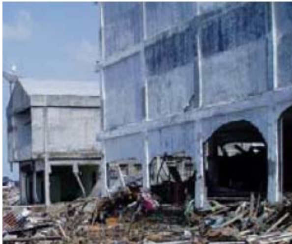
Figure 23. Confined masonry buildings in Banda Aceh, Indonesia, after the 2004 Great Sumatra earthquake and Indian Ocean tsunami 11 : good performance of confined masonry in the midst of devastation (top), and tsunami-induced out-of-plane failure of masonry walls at the ground floor level (bottom).
